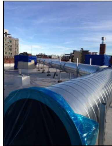
Dorm ERV Ductwork on the Roof
